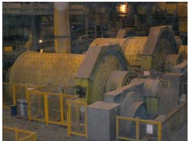
Fig. 1 - Existing 6.6kV 2MW Synchronous Motors
